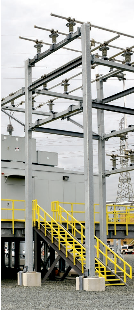
Switching station, Sewaren, NJ
